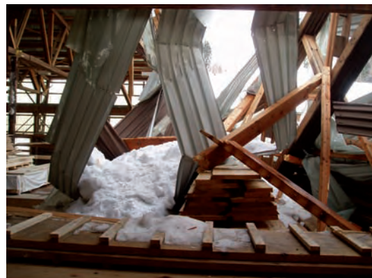
Figure 4: Snow pressure caused the collapse of a hall roof, Waldstatt 2006. (Source: Thomas Egli)
